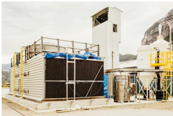
Carbon dioxide is captured within the plant’s gas-liquid contactor, which is essentially a repurposed cooling tower. An alkaline solution in the contactor reacts with acidic carbon dioxide in air to enrich the capture solution with potassium carbonate.
